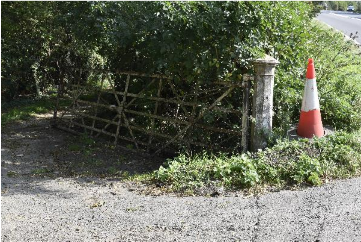
Photo 10 Cast iron gate pier and steel gate immediately north of the existing A47
